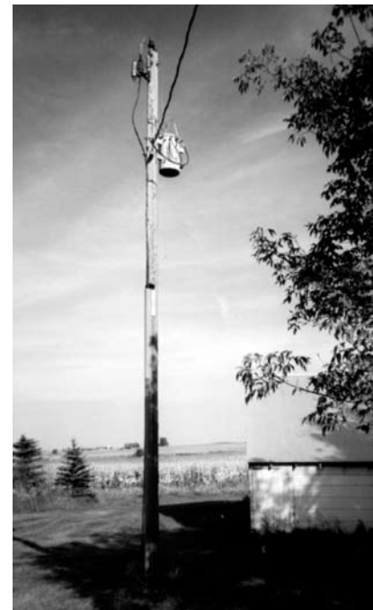
15 kV transformer with streak of rust on both sides – needs to be upgraded.
