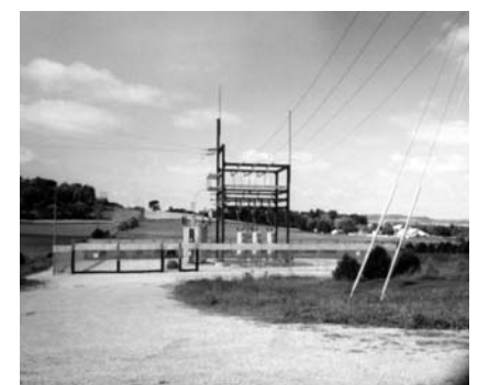
Newly constructed substation heavily grounded
