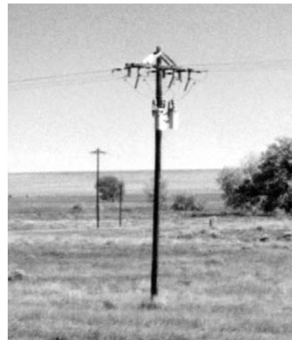
Three transformers altering current on a lateral
