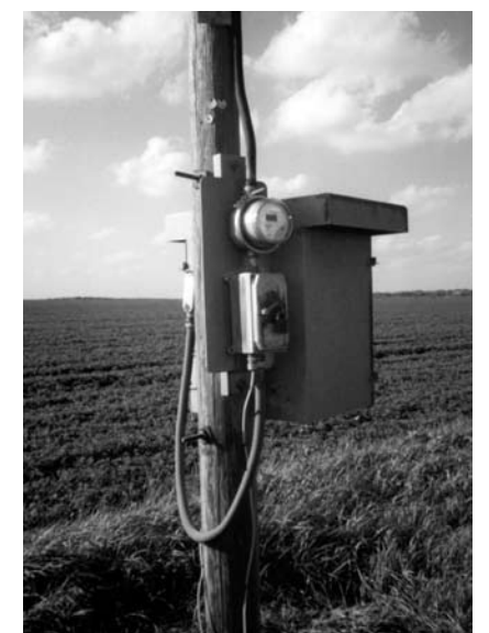
Cathodic system in northern Wisconsin
