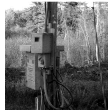
Cathodic system charging pipeline in Wisconsin
