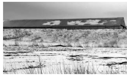
Rusty streaks became evident within just a few months after this barn was built.
