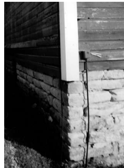
Phone entrance with ground going around barn, splicing into the barns electrical grounding wire.
