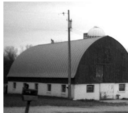
Transformer located right next to the barn – bad location!
