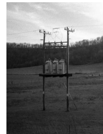
Bank of three capacitors.
