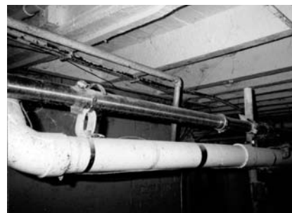
Milk pipelines are part of the electrical grid on your farm.
