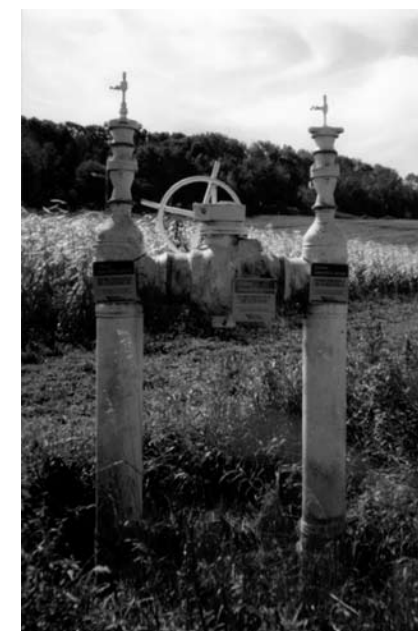
Gas pipeline shut-off
