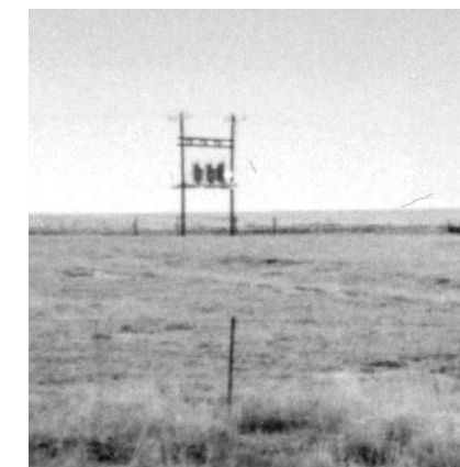
Bank of three capacitors.
