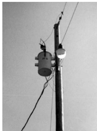
27.5 kV transformer running properly. 35s are being seen more often in replacements.
