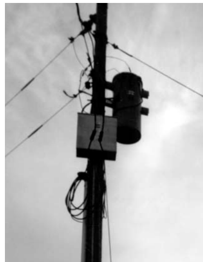
Totally rusted little 15 kV transformer running hot and rusty.
