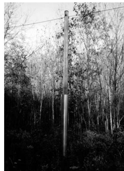
Twenty poles very close together, some with metal collars inducting current onto gas pipeline.
