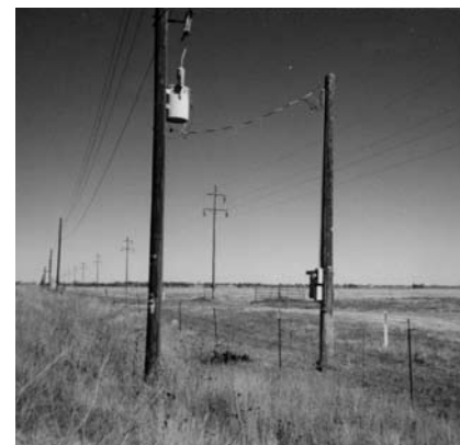
Two electrical transmission lines running parallel with gas line – see transformer with meter cathodically inducing charge onto pipe (Colorado).
